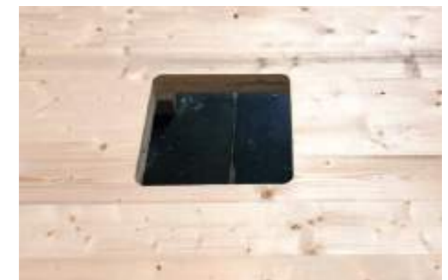
Cut-out, residual radii not removed
